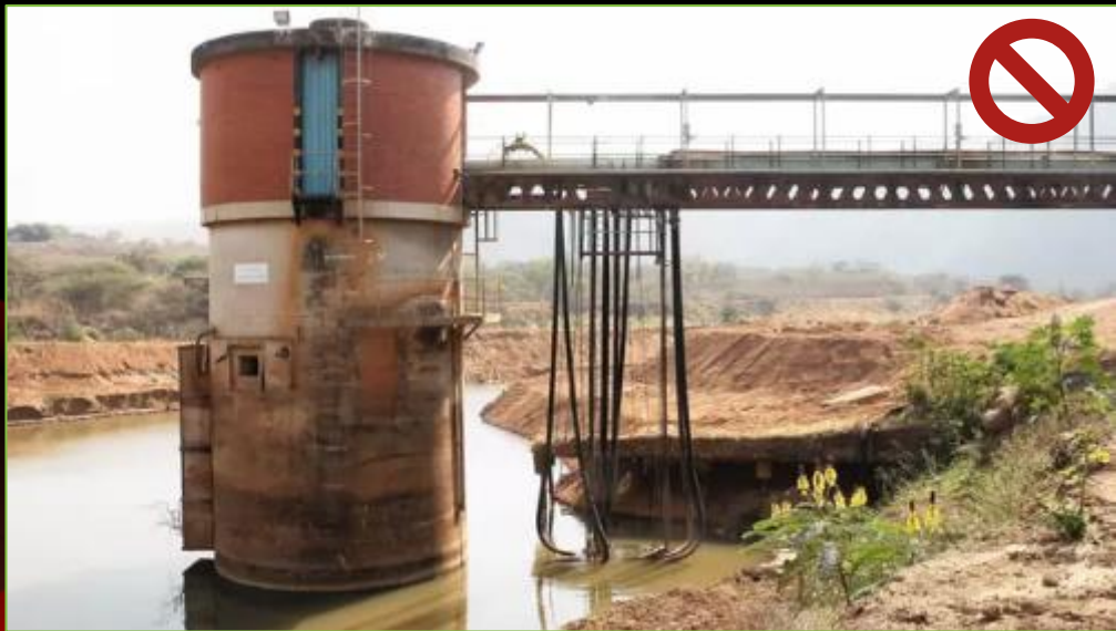
A: Neglected Water Treatment Works
